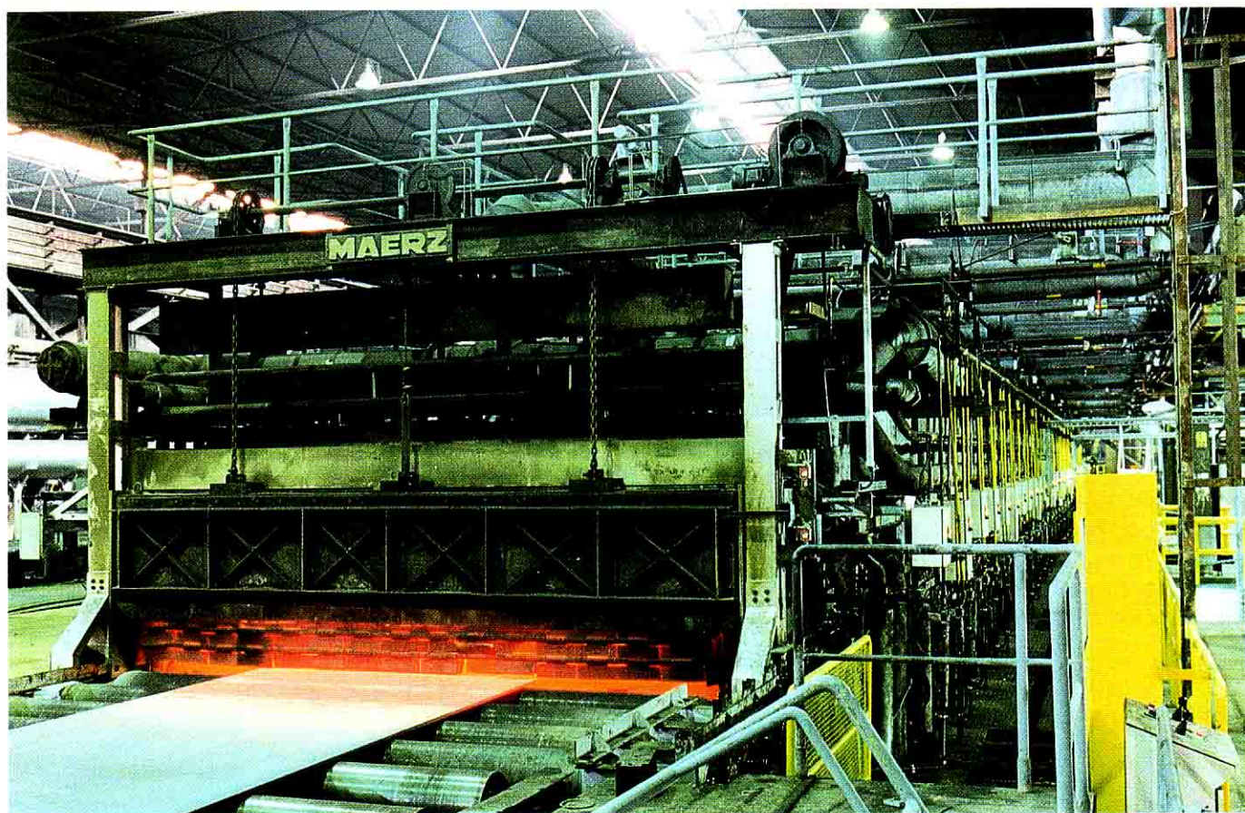
Fig.23: Heating oven line with roller conveyors, total length 114 m
